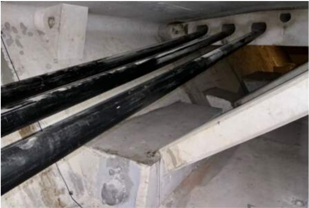
Figure 8: Obstacles around ducts
