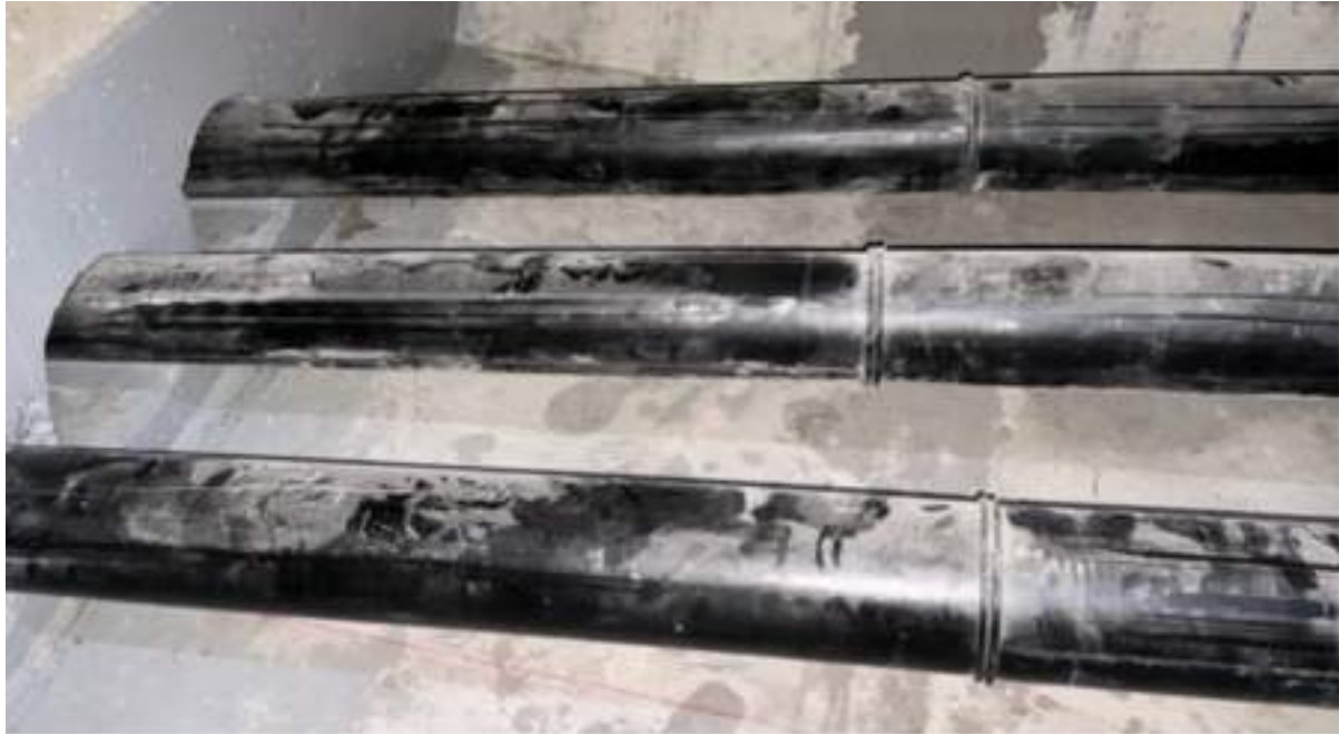
Figure 7: Anchorage and welding joints blockers
