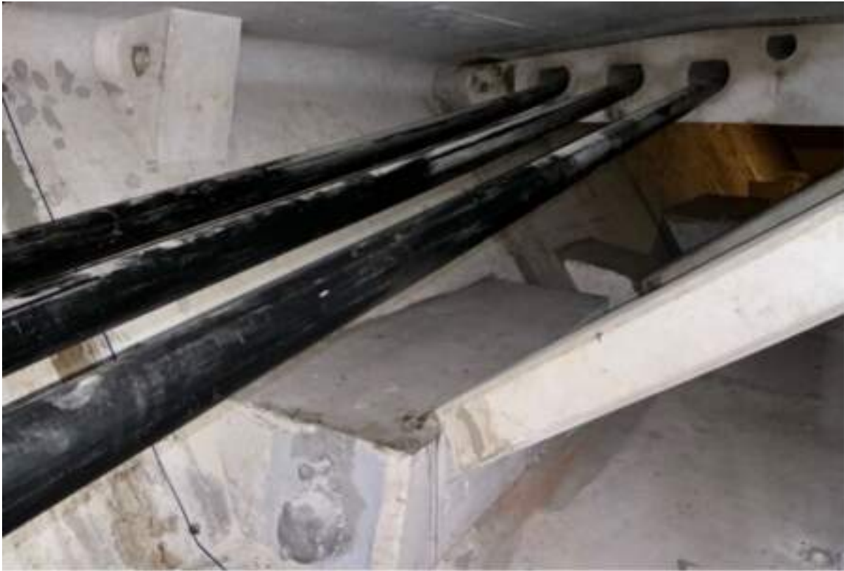
Figure 8: Obstacles around ducts
