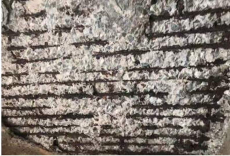
Rusting and peeling areas (front plate)
