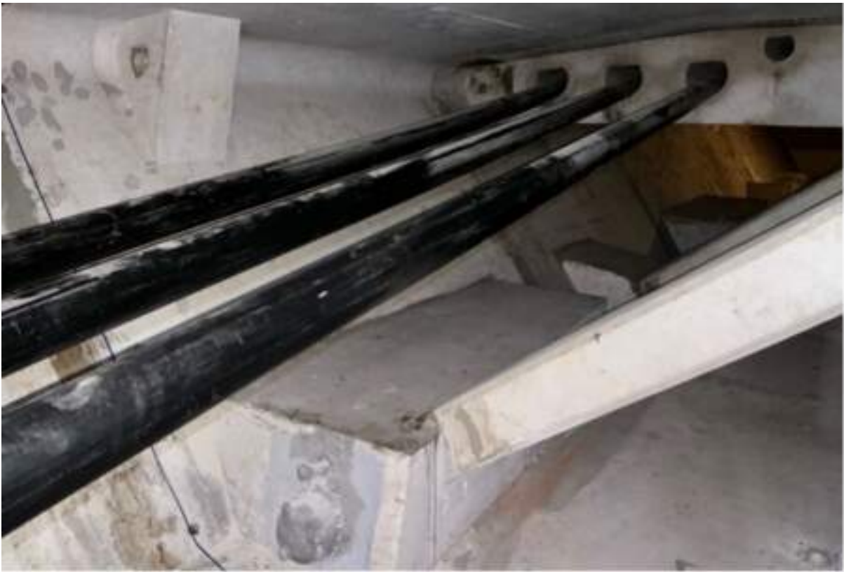
Figure 8: Obstacles around ducts
