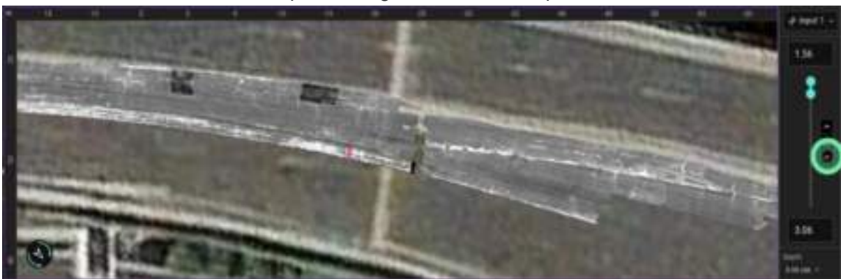
Figure 5. Major surface defects at asphalt layer (cracks)
