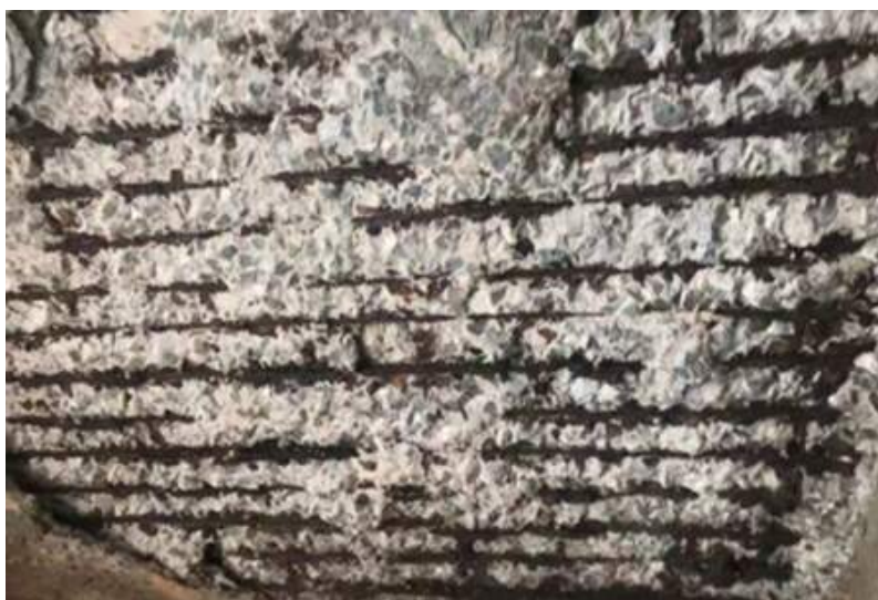
Rusting and peeling areas (front plate)
